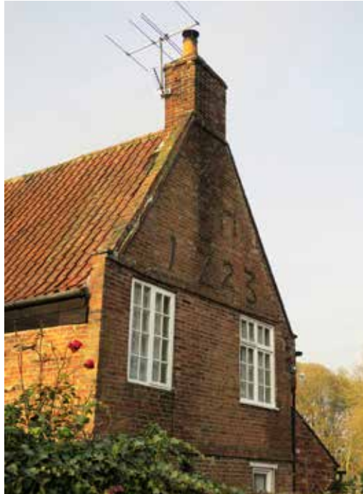
Figure 35: Clay pantile roof, parapet gable with internal gable-end stacks ©Bottesford Parish Council, 2019.
