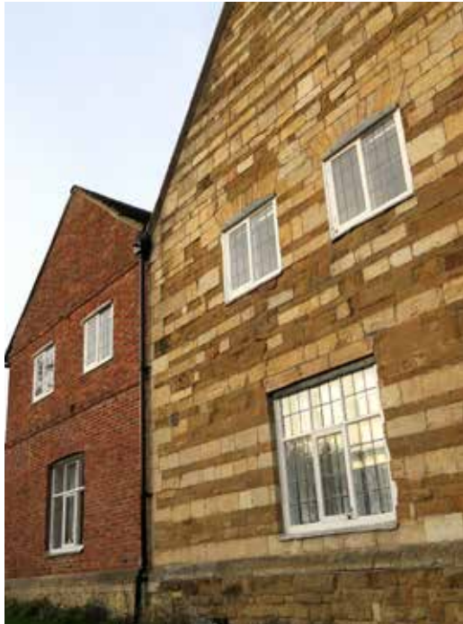
Figure 39: Side elevations with alternating ironstone and sandstone courses (right) and red brick (left).
