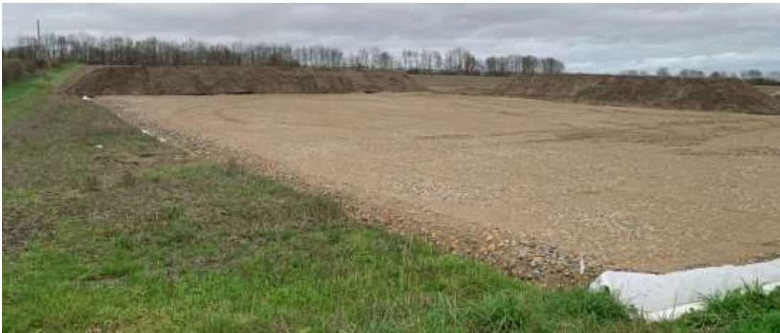
Location: Elsham-Lincoln Pipeline, 2023
