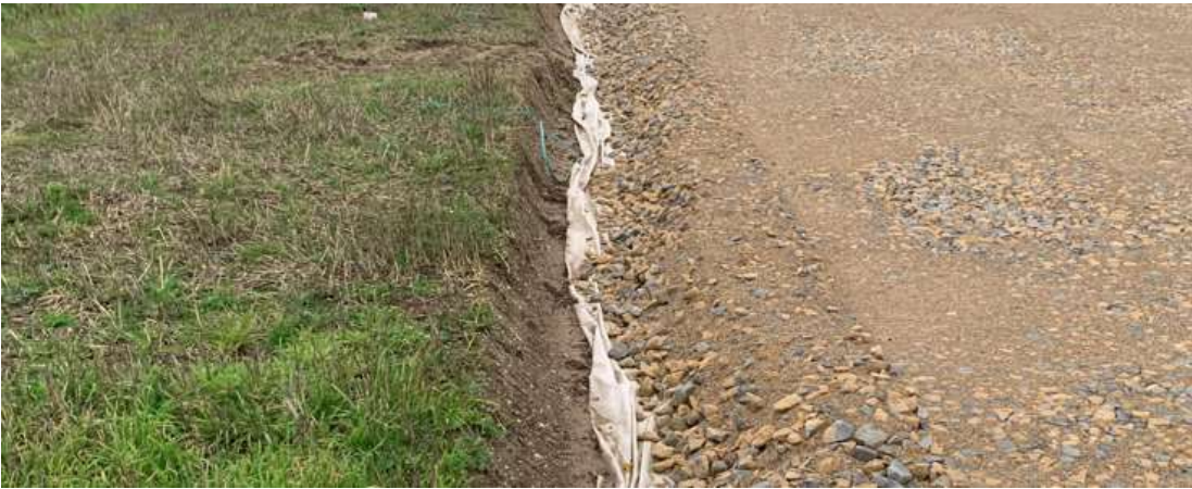
Location: Elsham-Lincoln Pipeline, 2023
